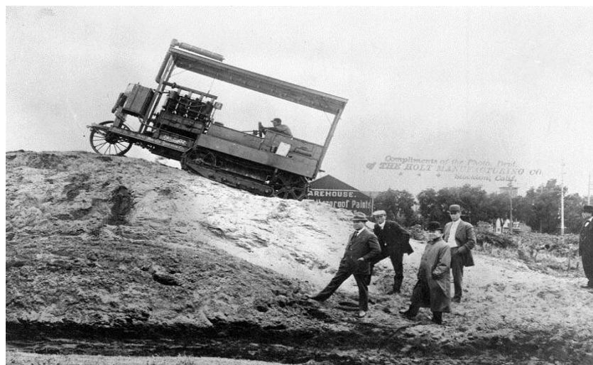
The first Caterpillar tractors were used to help build the Aqueduct photo credit: Water and Power Associates
